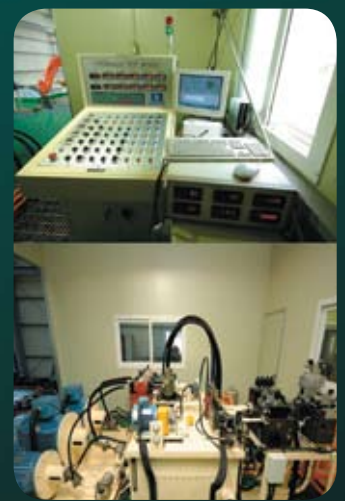
Control console with monitoring panel Power pack to replicate actual situation
